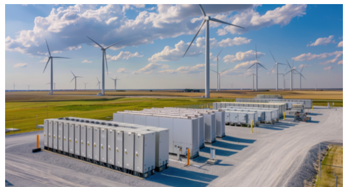
Figure 1: Containerised battery systems (Source: Avnet Silica)
